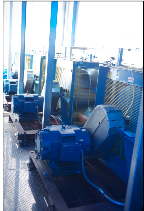
figure2. four 50,000CFM air-handlers on 5th floor mechanical space
